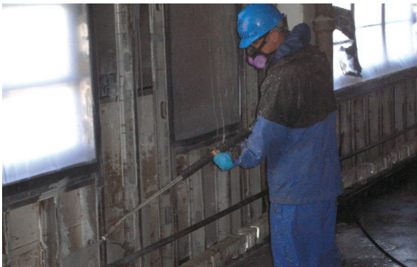
Workers use Fiberlock's ShockWave disinfectant/sanitizer to treat mold in a building affected by recent hurricane damage.
