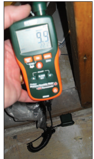
Figure 5: Use of a penetrating (pin-type) moisture meter to verify that wood frame has a water content of less than 15 percent
