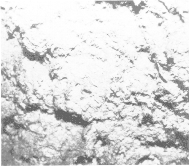
Friable, fluffy sprayed-on material
