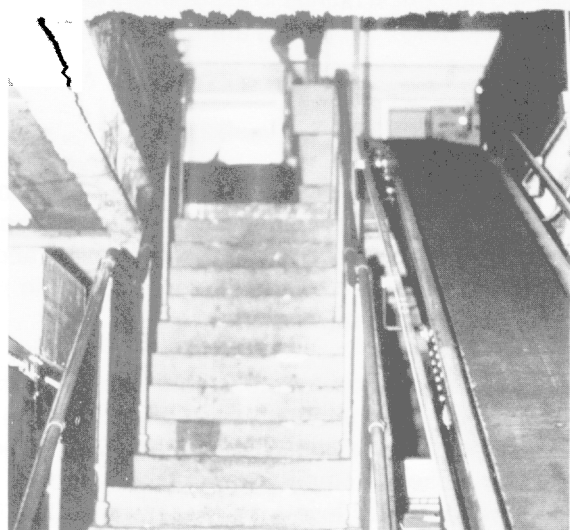
High activity level near friable asbestos
